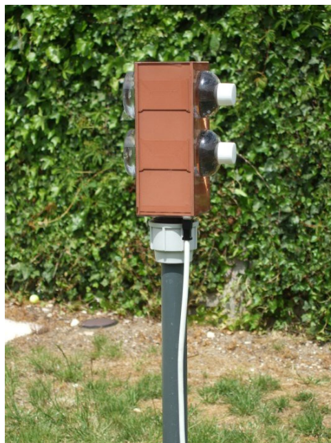
Figure 4. Sensor installed on 32mm OD PVC pipe approx. 1m above ground
